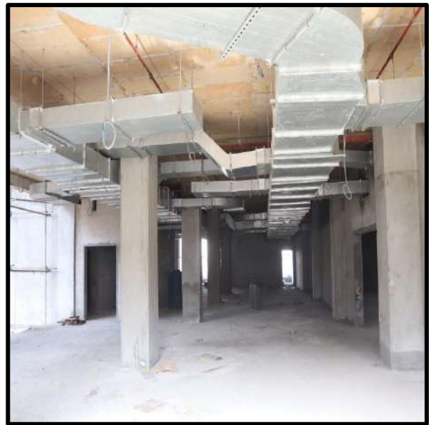
Picture 99: HVAC Ducting of PLGA Lahore
