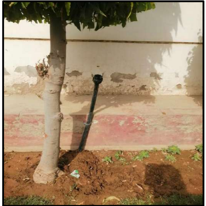
Picture 16: View of the Consumer House connection
