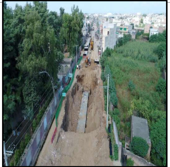
Picture 68: Conduits laying is in progress near Technical College Site 2 Marala Road Sialkot
